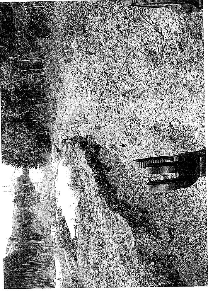
Easton Ridge Road April-09 Damaged from Runoff near proposed rezoning.
